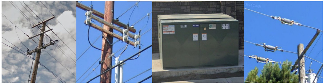
Figure 3 - (L-R), Gang Operated (pole mount), Hook Operated, Gang Operated (pad mount), In-Line
